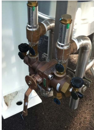
Figure 4 Example of pressure safety valves on a static storage tank
