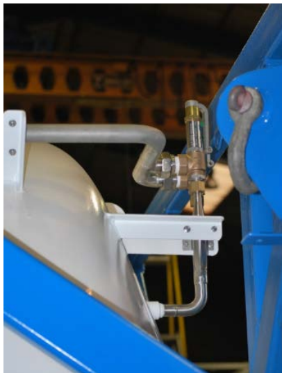
Figure 2 Example of vent manifold on a portable tank
