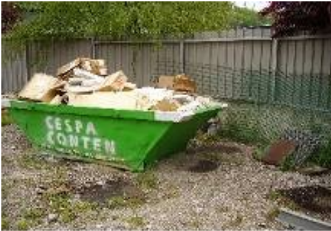
Figure 3 Overloaded container in incorrect area
