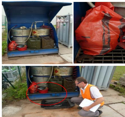
Figure 1: Drums in containment with additional drip tray and absorbent material to hand.
