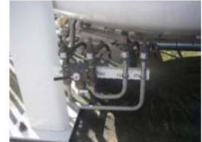
Typical tank relief valves
