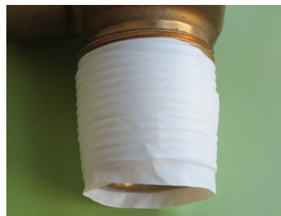
Figure 3 Typical example of excessive PTFE tape applied to the valve inlet thread
